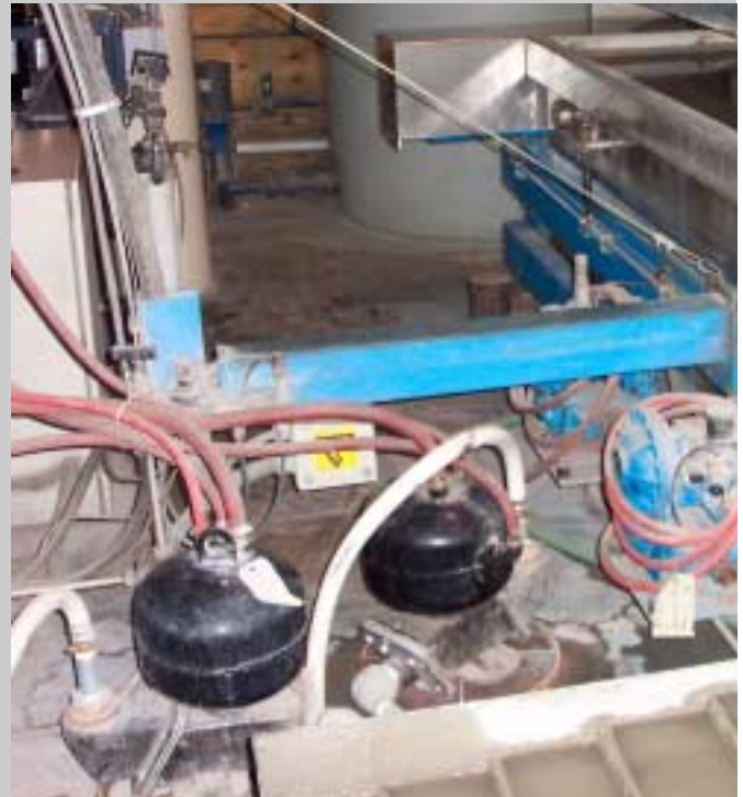
2 of the PITBULLS® (black) at 1 year inspection - May 2006 2 of the AODD pumps that were replaced (blue) are sitting off to the right.
